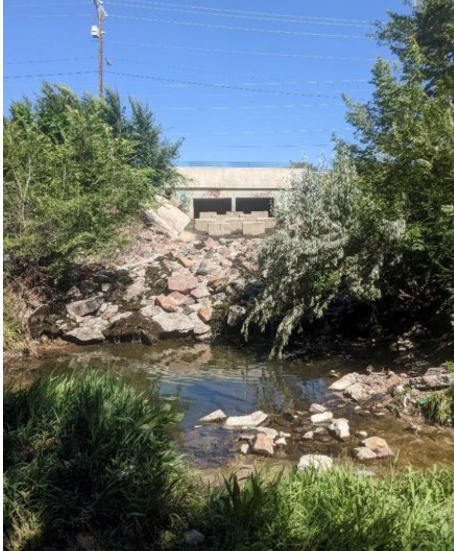
Figure 8: Box culvert on east side of Reach 2. Water consists mainly of urban wasted water. (Date: 2022)
