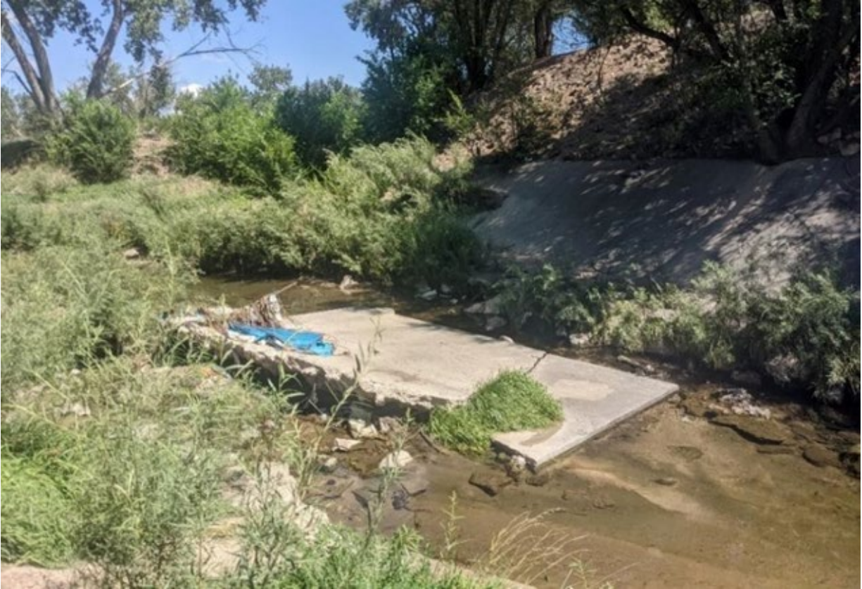
Figure 9: Reach 3 - South Channel image showing the hardening structures along the bank and a piece that has fallen into the stream channel. (Date: Aug 2022).
