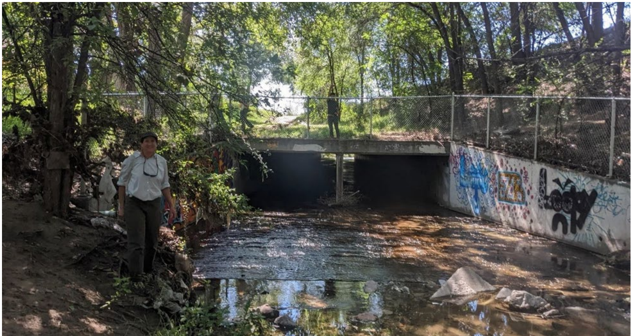
Figure 3: Box culvert on south end of Reach 1 under Pikes Peak Road. Image is taken facing south. Notice the steep bank on the right (west) side of the photo. (Date: 2022).
